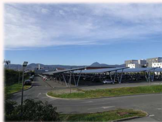
Ombrières CHU Estaing – Clermont-Ferrand
